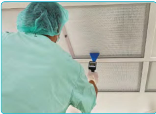
HEPA Integrity Test
